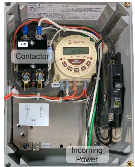
Figure 2: Disconnect Control Panel
