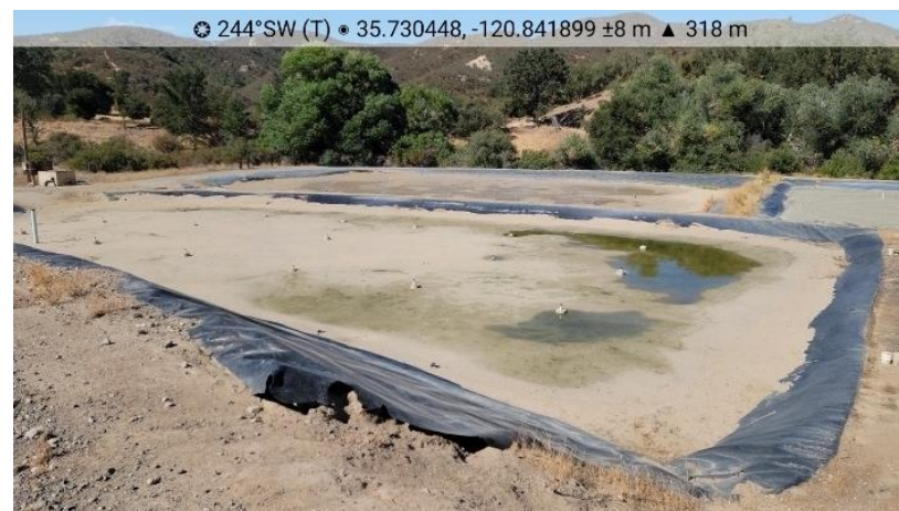
Photograph 4. Existing Sand Filters at Spray Field, Facing Southwest.
