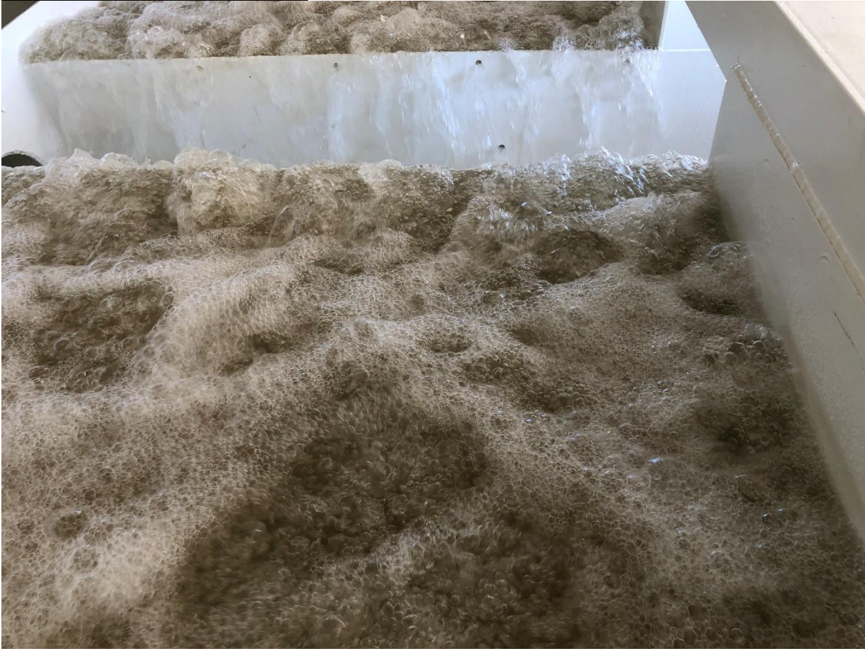
One of Many Backwash Cycles
