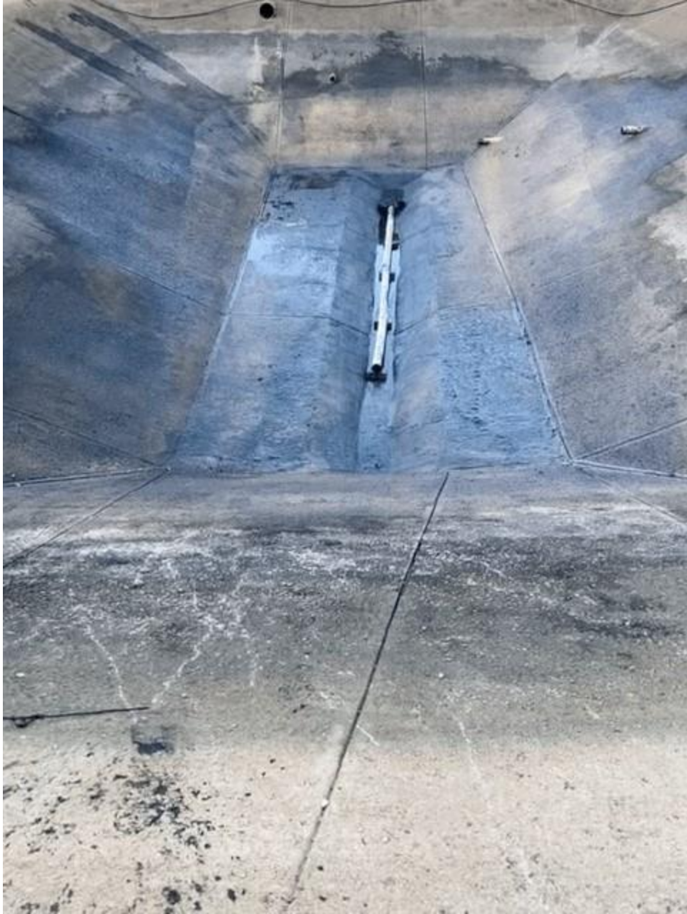
BACK WASH RECOVERY BASIN EMPTY
