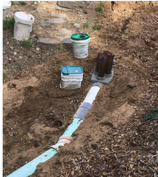
Figure 10 Existing Dechlorination Point
