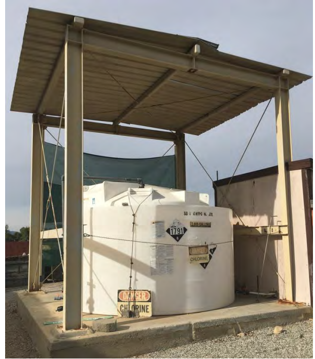
Figure 6 Existing Disinfection Facility
