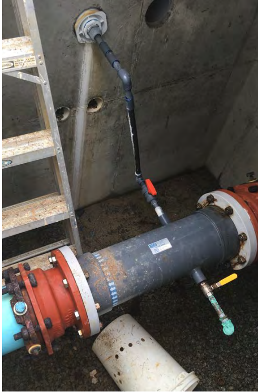
Figure 22 Existing Effluent Chlorination Dosing Point
