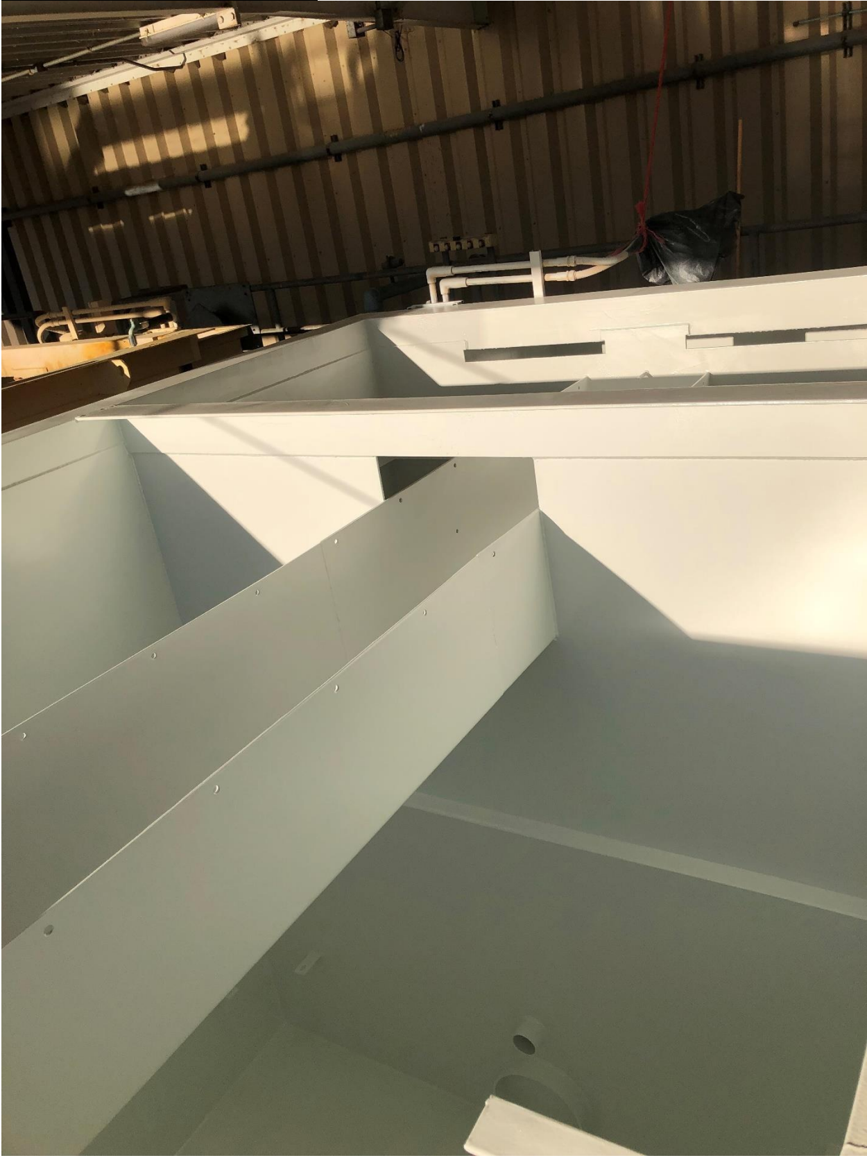
Filter #3 Painted - Looking West
