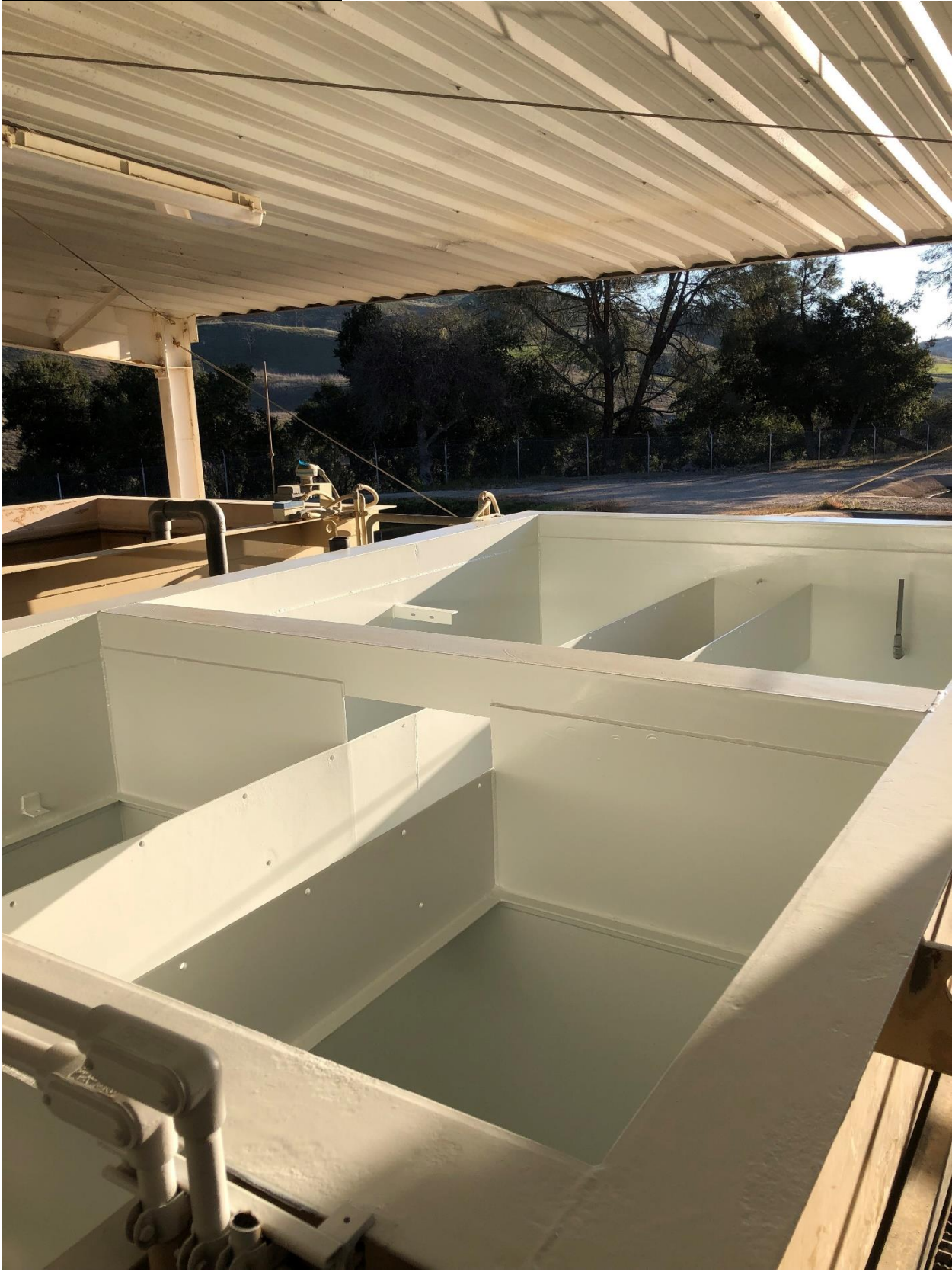
Filter #3 Painted - Looking East
