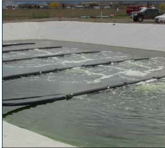
Figure 3-1: In-pond Extended Aeration Chains
